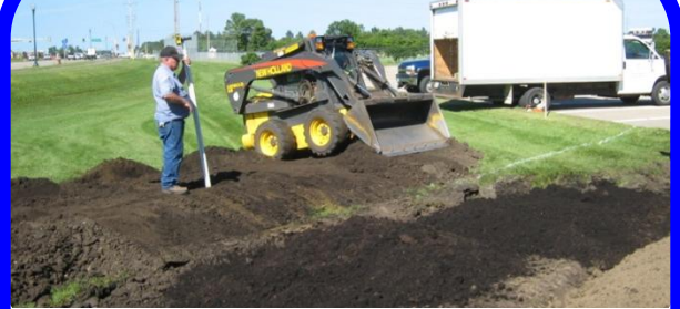
The bioretention cells were over-excavated to provide soil to build the confining perimeter berms.
